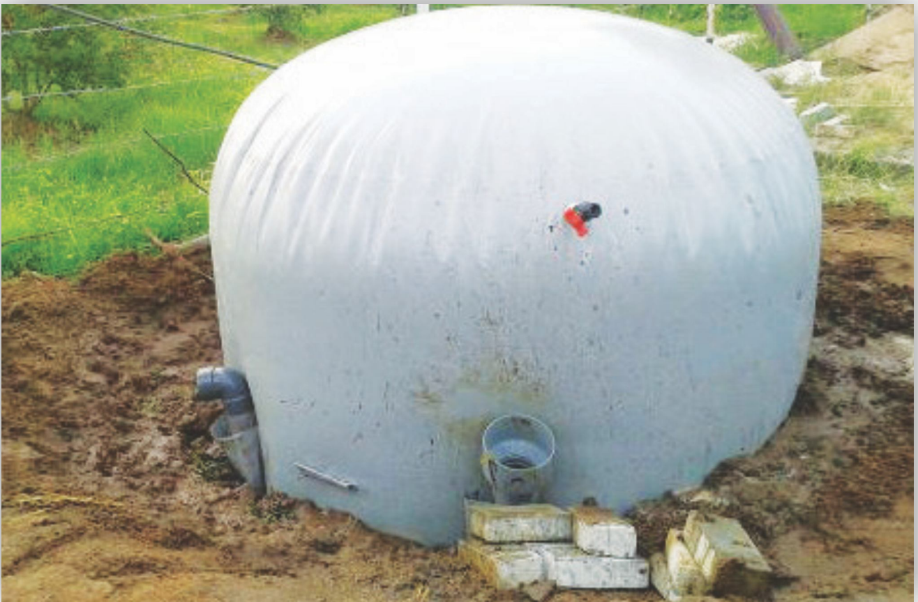
Bio Gas Plant
